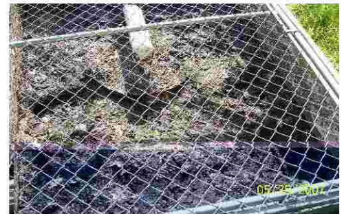
Plugged Up Sand Filter
